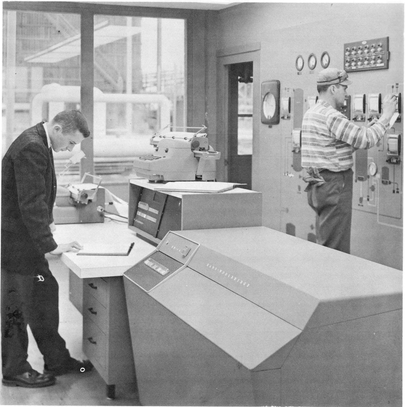
Here is an RW-300 Computer Control System installed in the B. F. Goodrich Chemical Company plant at Calvert City, Kentucky. The RW-300 Digital Control Computer is in the foreground, the operator's console with input-output typewriters, and a conventional graphic panel. The system automatically reads instruments in the plant, prints out operating variables and calculated values, and controls a unit producing vinyl chloride monomer as well as a near-by acrylonitrile unit. (Figure 41)
