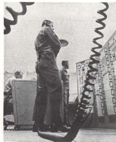
SIMULATOR installed by ACF Electronics at Vandenberg AFB, Calif., is used to train Titan II launch control center crews
