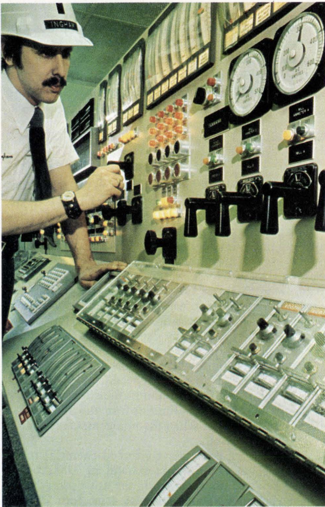
Powerhouse. Control console for computer-controlled boiler system at Buick Motor division's Flint, Mich., plant logs boiler data every hour and alerts operator any time conditions become unsafe.
