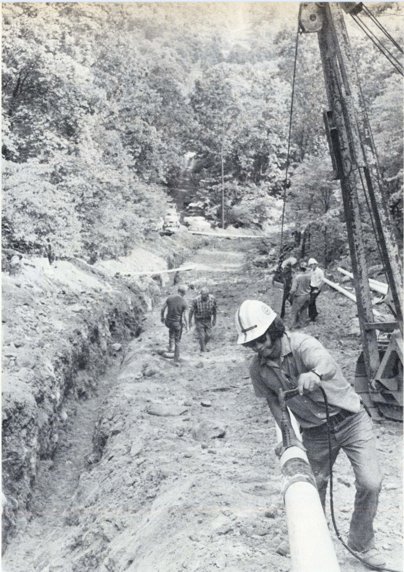
Buried waveguide. AT&T is installing a 20-mile test link of cylindrical millimeter waveguide in northern New Jersey. The waveguide eventually will carry up to 500,000 telephone conversations in a frequency range from 40 to 110 MHz. Actual operation will begin in the 1980s.
