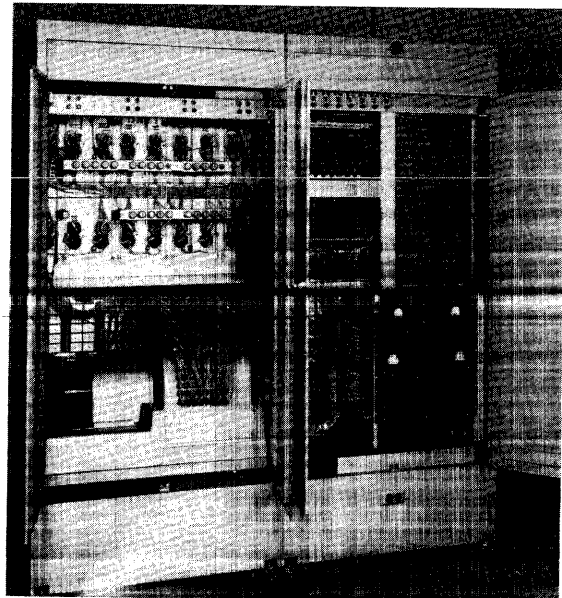
Fig. 7. Rear view of Speed Tally Central Equipment
