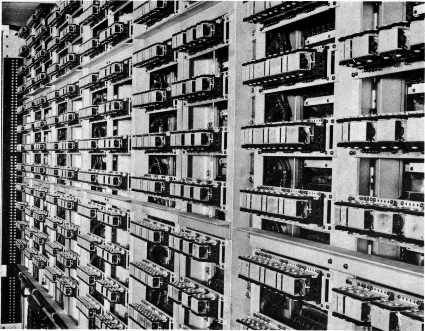
X Storage Counter Relays
